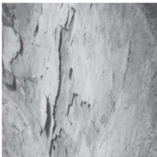
Fig. 2. corrosion products in the interior surface of stack
